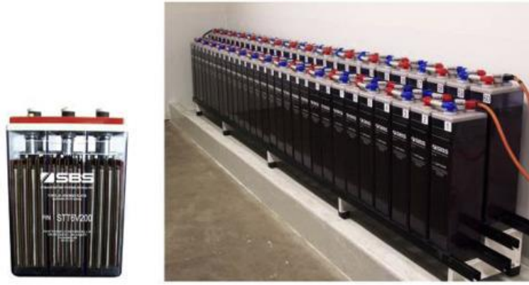
Figure 2.3.6 : Lead Acid Battery
